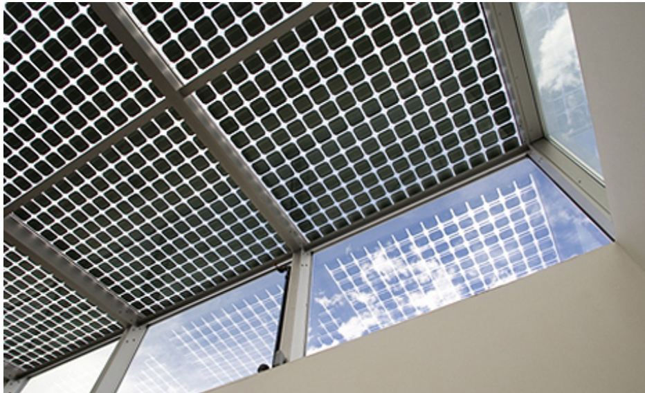
Figure 13: Solar glazed Building Integrated Photovoltaics.
